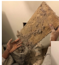
Actual Debris From Lakeside Common Elements Dryer Vent Shaft
